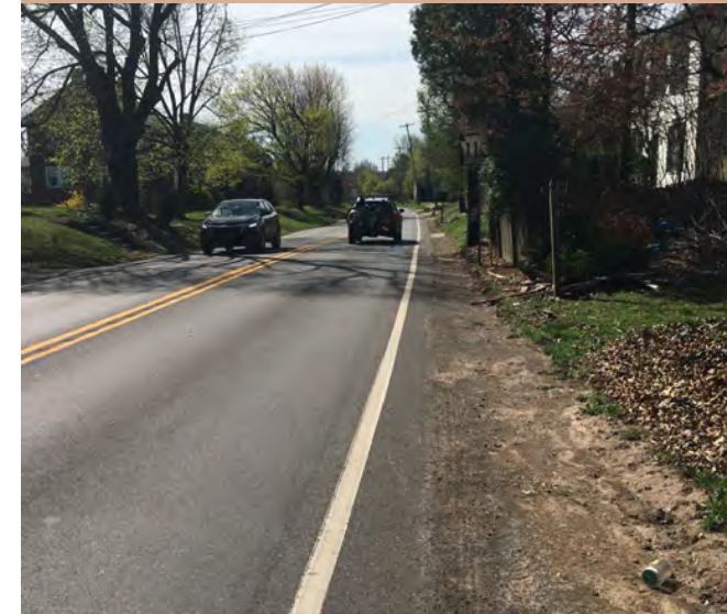
Limited shoulder along PA 113 south of village
